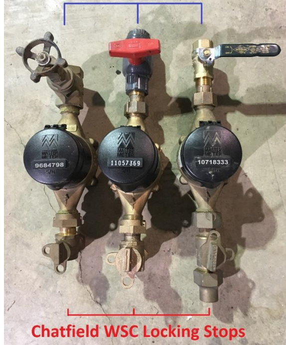
Customer Installed Shut Offs
